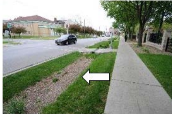
Photo 14-2. Bioswale treated with herbicide accidentally. Vegetation is sparse, which may allow erosion. Consider reseeding or replanting and providing adequate signage in English and Spanish to ensure the practice is not continually treated with herbicide. (Credit: EPA Region 5)
