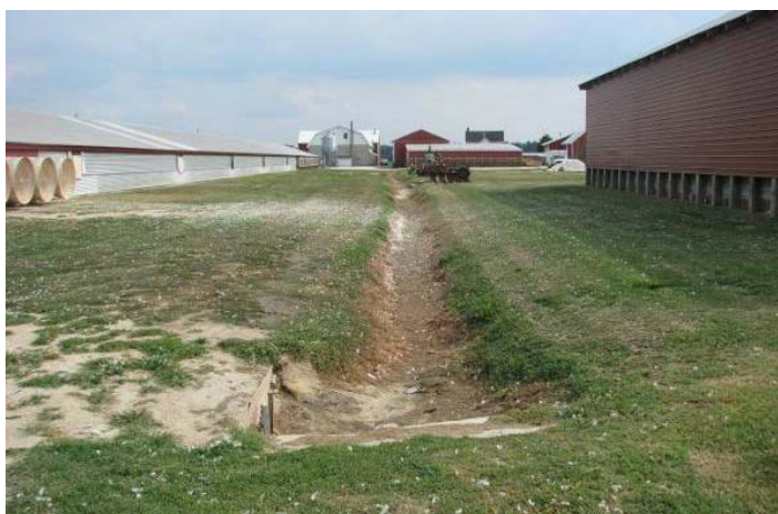
Photo 17-7. A poultry operation designed to have precipitation drain away from houses would discharge if contaminated runoff enters a water of the United States. (Source: EPA Region 3)
