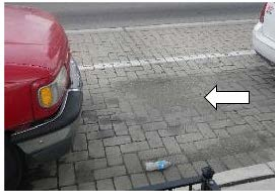
Photo 14-8. Visible silt on the permeable pavement surface, indicates that water is collecting before infiltrating. Maintenance, such as sweeping or vacuuming is needed. (Credit: EPA Region 5)
