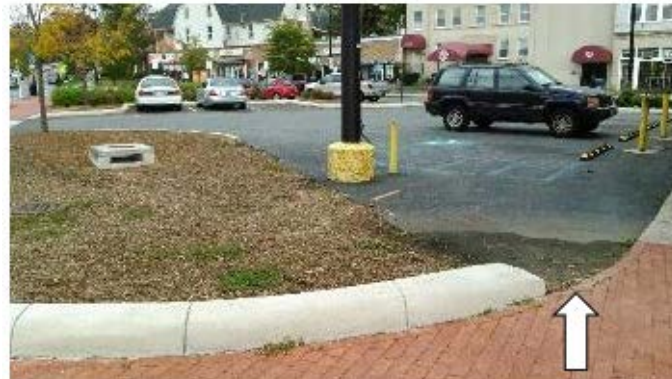
Photo 14-3. Inappropriate grading is another common design flaw in infiltration-based control practices. If a parking lot, street or other impervious surface is not properly graded towards the control or is bypassing the control, the BMP is not serving its intended purpose. In the photo above, the wet spot on the pavement indicates either poor grading in the installation or poor drainage by the control. Consider adjusting the grade. (Credit: EPA Region 5)
