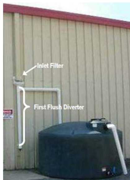
Exhibit 14-10. First Flush Diverter (Credit: NCSU BAE)
