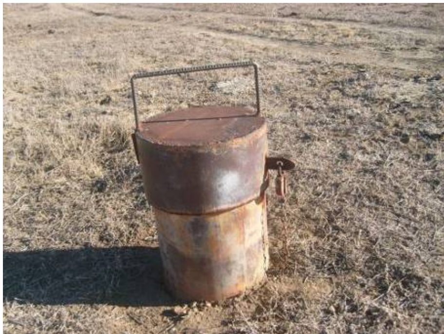
Photo 2. Well head at north end of site along fence running north-south
