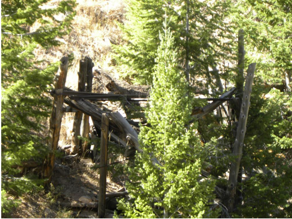
Photo 5. Wood frame debris
