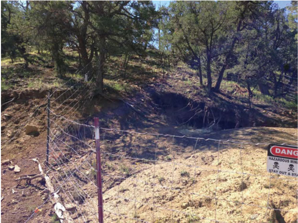
PHOTO 2: View from the southwest of adit fencing, showing portion of fence to be re-stretched.
