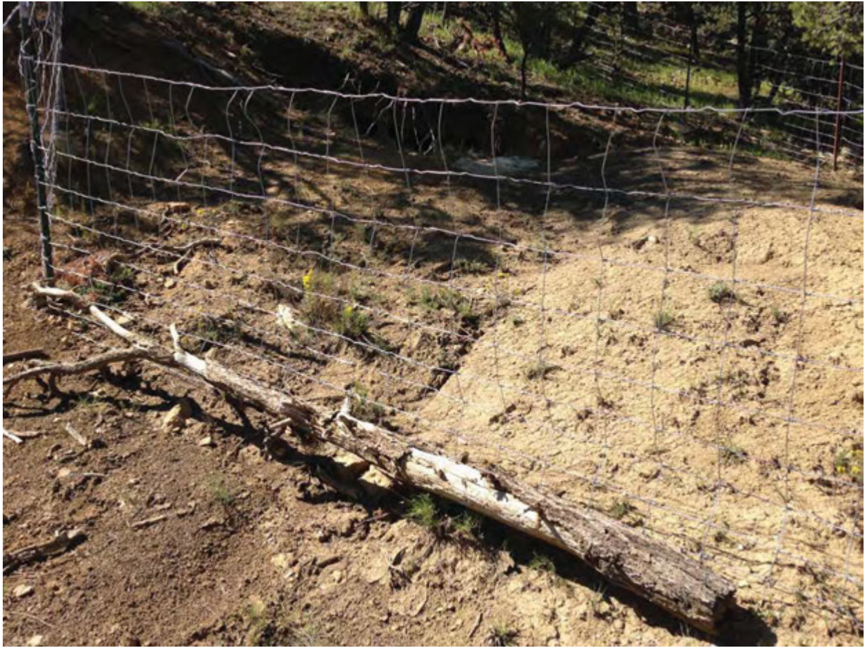
PHOTO 4: View of the adit from the southwest showing fencing to be re-stretched.
