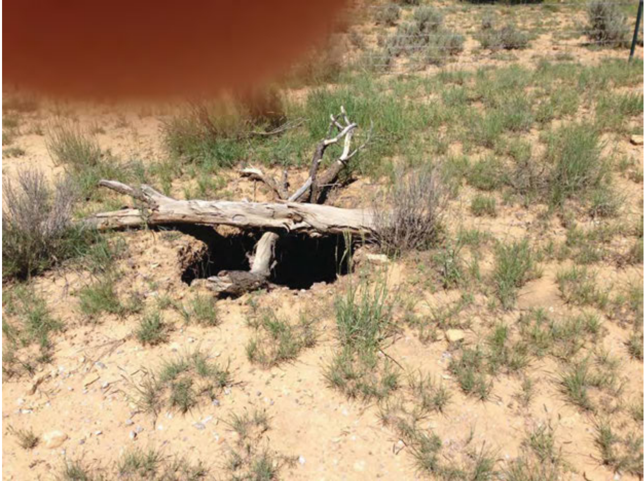
PHOTO 3: View of the opening that is apparent in the Ruby 3 former shaft entrance.
