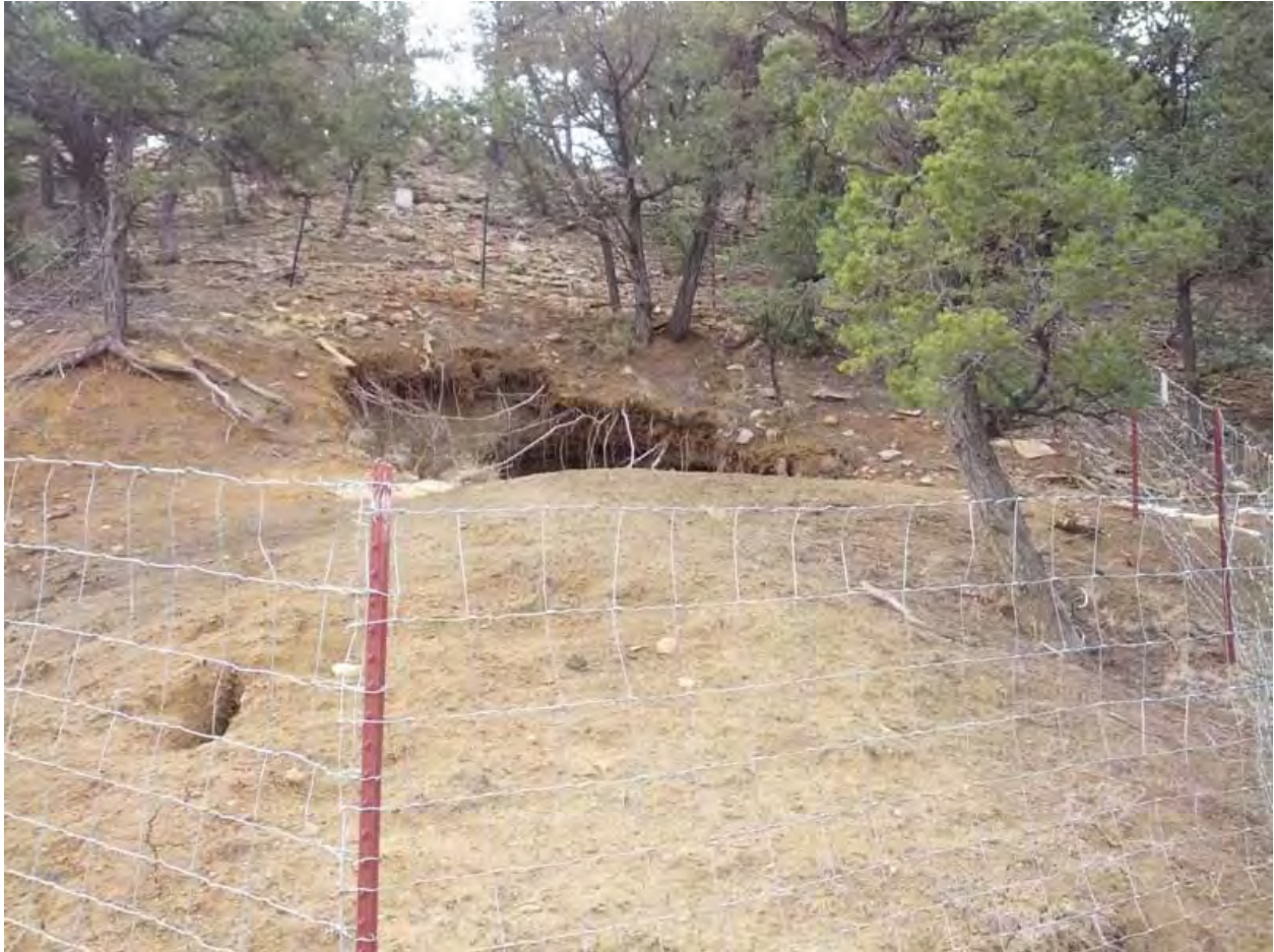
PHOTO 3: Ruby Mine #1 Adit opening and fencing, facing east. Note field fencing and no barbed wire.
