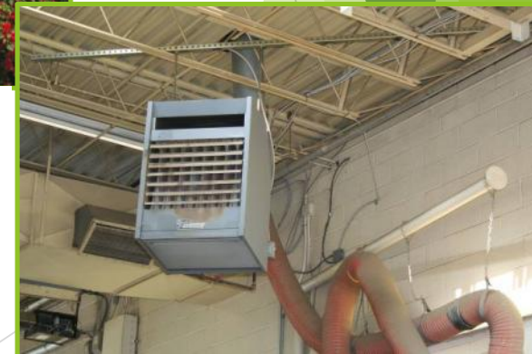
Infrared Heater - Lorton, VA
