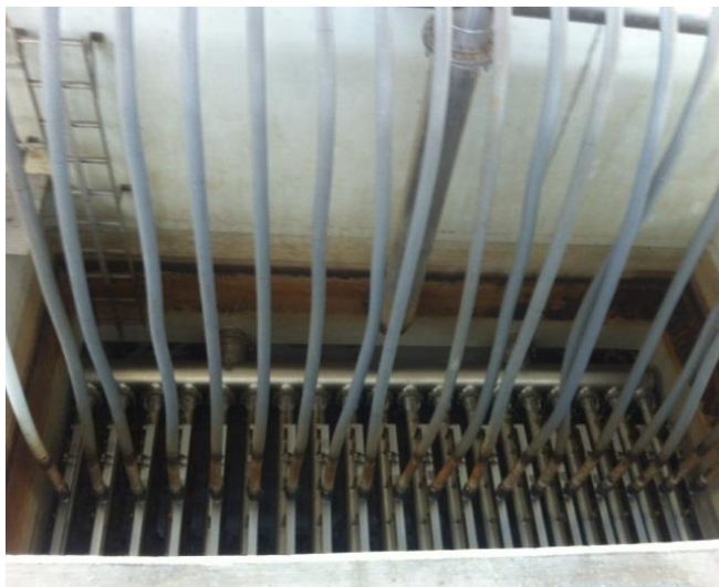
Figure 6-2. Submerged MF membranes at OCGWR
