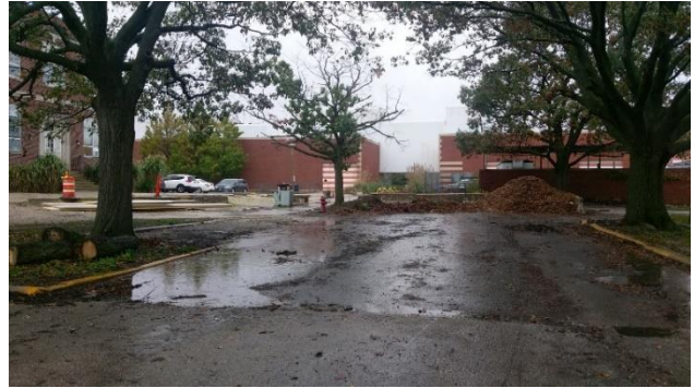
Figure 1 shows standing water and other debris in the westmost section of parking lot F4.
