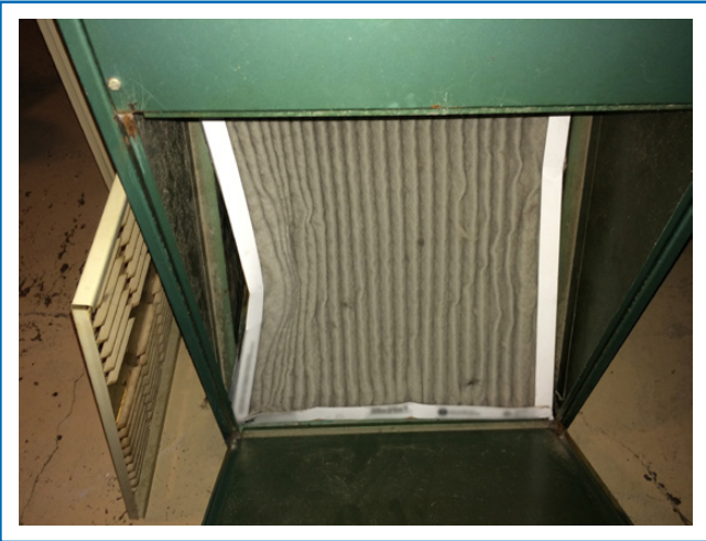
Figure 8. Example of large amounts of bypass airflow around a filter in an air-handling unit because of improper installation combined with excessive loading that increased the pressure drop across the filter beyond what the filter was capable of supporting. Photo credit: Brent Stephens.
