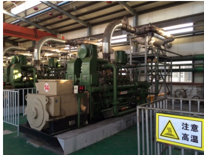
Power Plant with 500 kW Gensets
