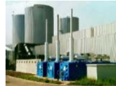
Combined Heat & Power
