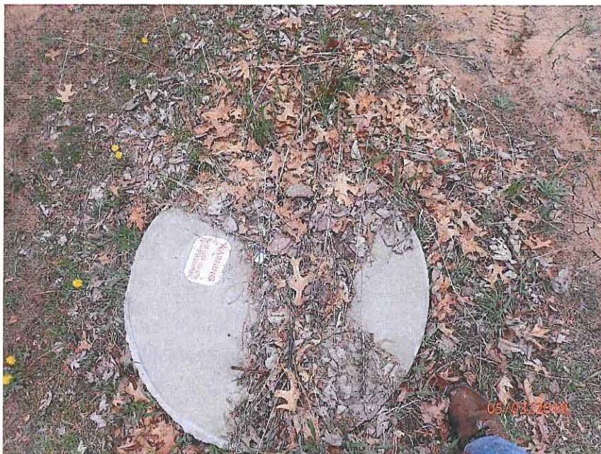
194: P5030102 Description: Septic Tank Location: SO4 Date/Time: May 3, 2018/12:17 PM
