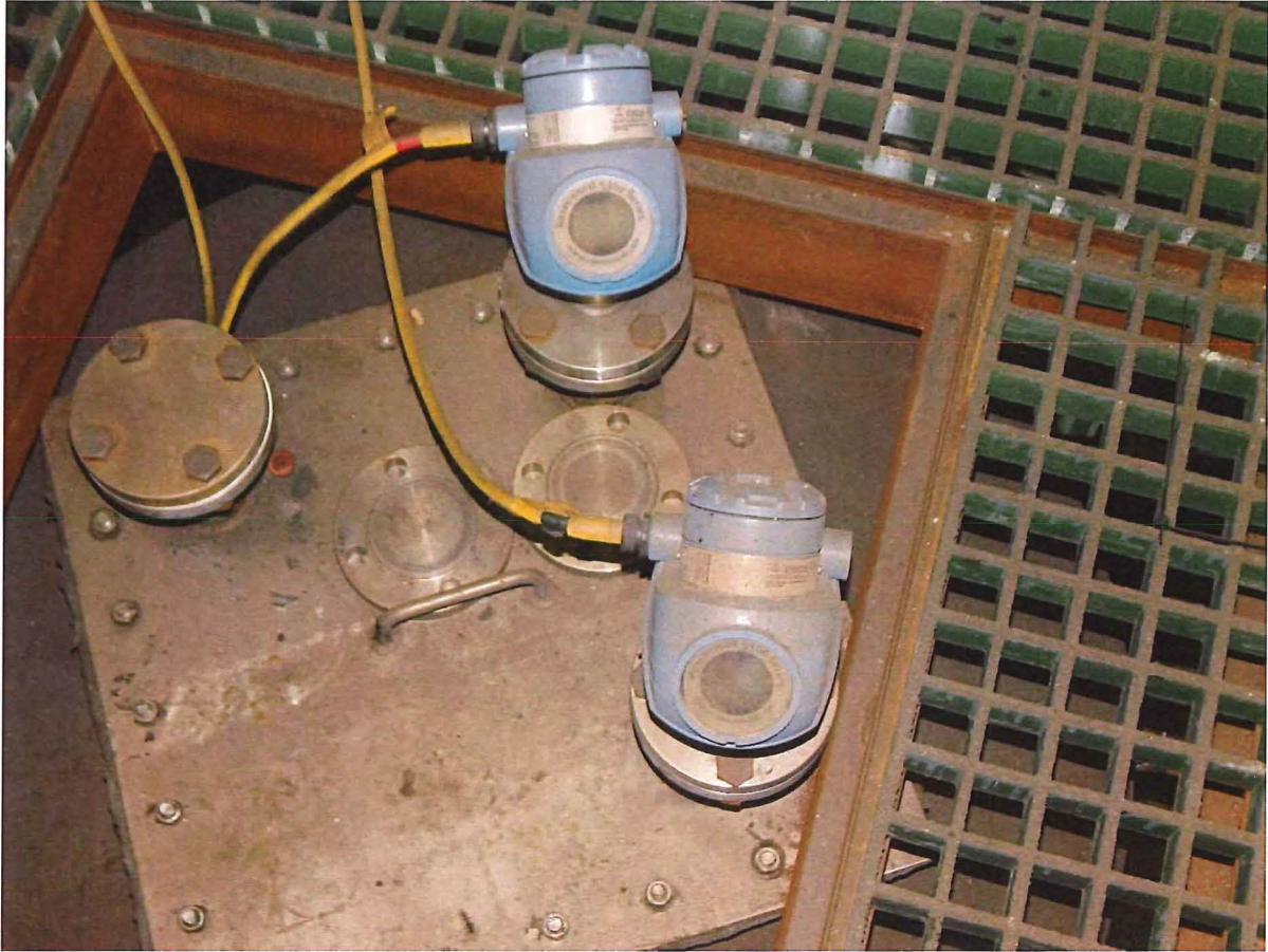
Picture 11: Chrome Line Evaporator: Picture of redundant level sensors installed on top of Evaporator
