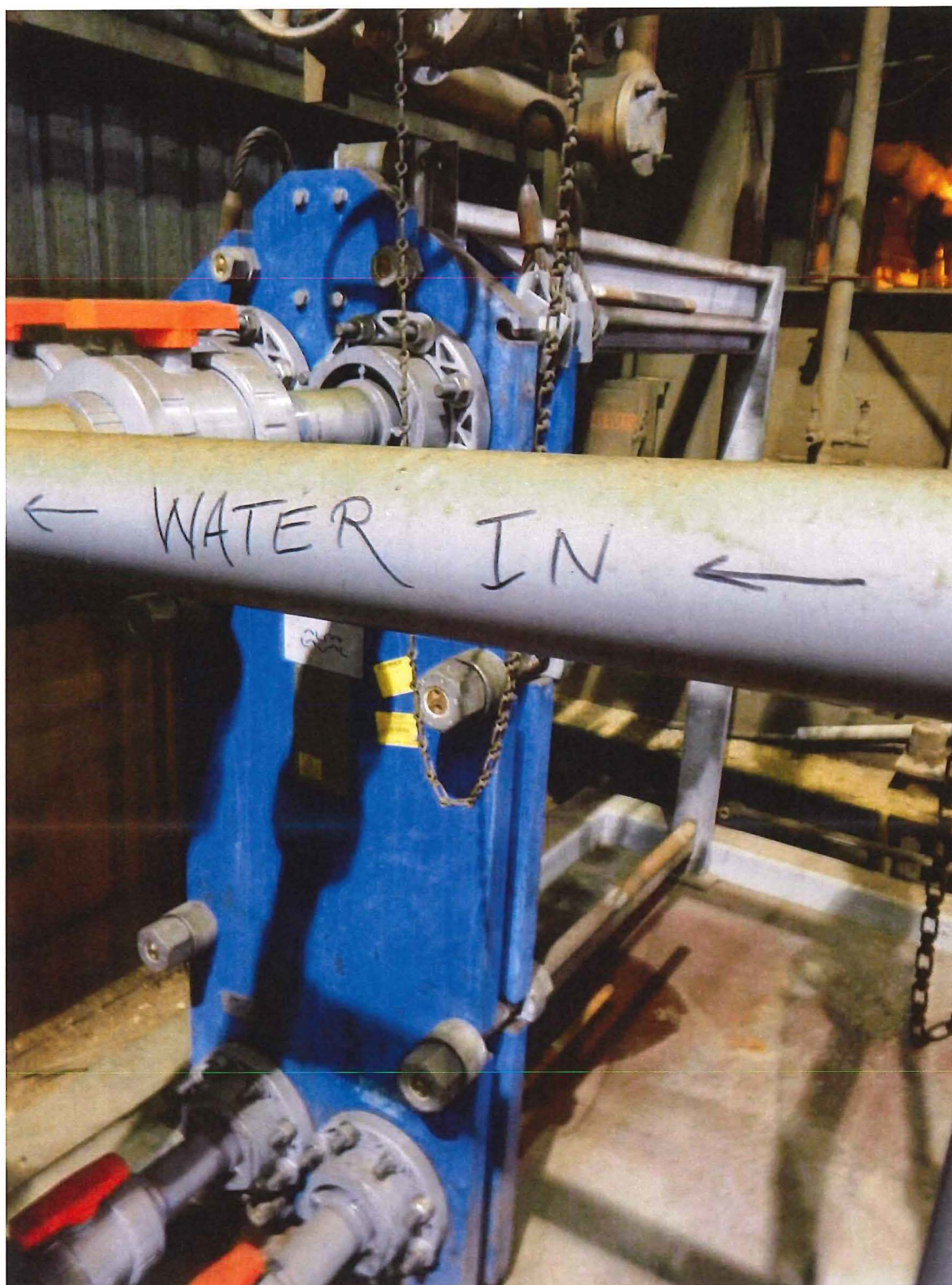
Picture 5: This picture shows the newly installed back up double walled heat exchanger pursuant to the Enhancend Wastewater Process Monitoring Design
