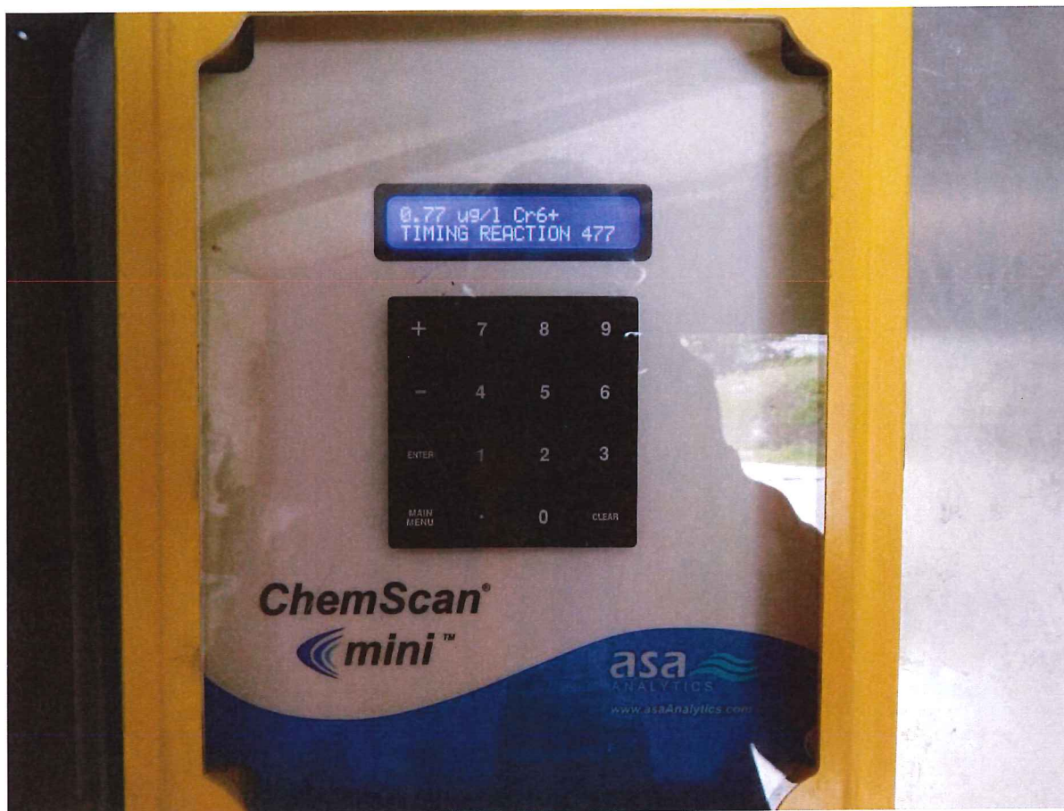
Picture 10: Final treatment plant discharge: Picture of ChemScan unit currently being trialed
