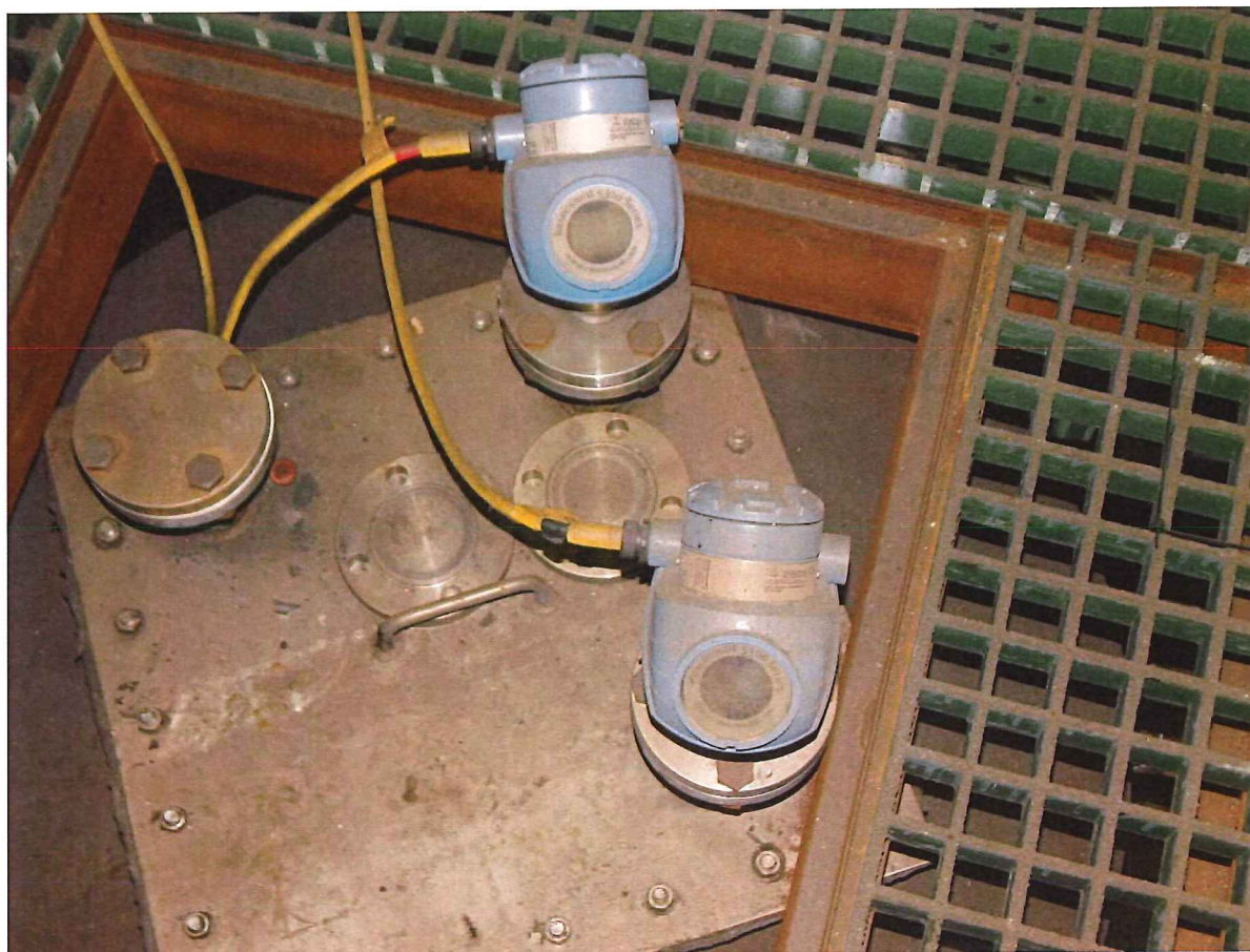
Picture 11: Chrome Line Evaporator: Picture of redundant level sensors installed on top of Evaporator
