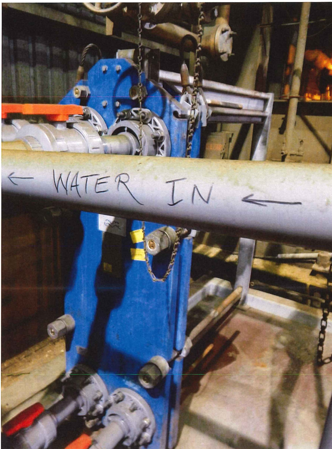
Picture 5: This picture shows the newly installed back up double walled heat exchanger pursuant to the Enhancend Wastewater Process Monitoring Design
