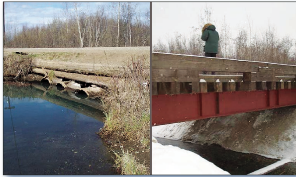
Figure 2. Partners replaced small culvert pipes (left) along Chena Slough with a new bridge (right) that allows the water to flow freely.
