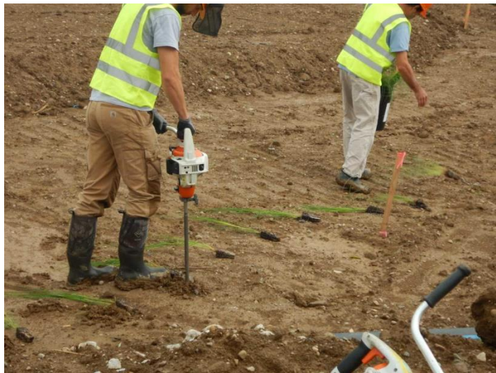
Emergent marsh habitat restoration has begun on-site. Here workers drill holes to plant vegetation. This type of habitat can be found on the edges of streams and lakes and provides a home or food source for a variety of fish, frogs, snakes, turtles, birds and mammals.
