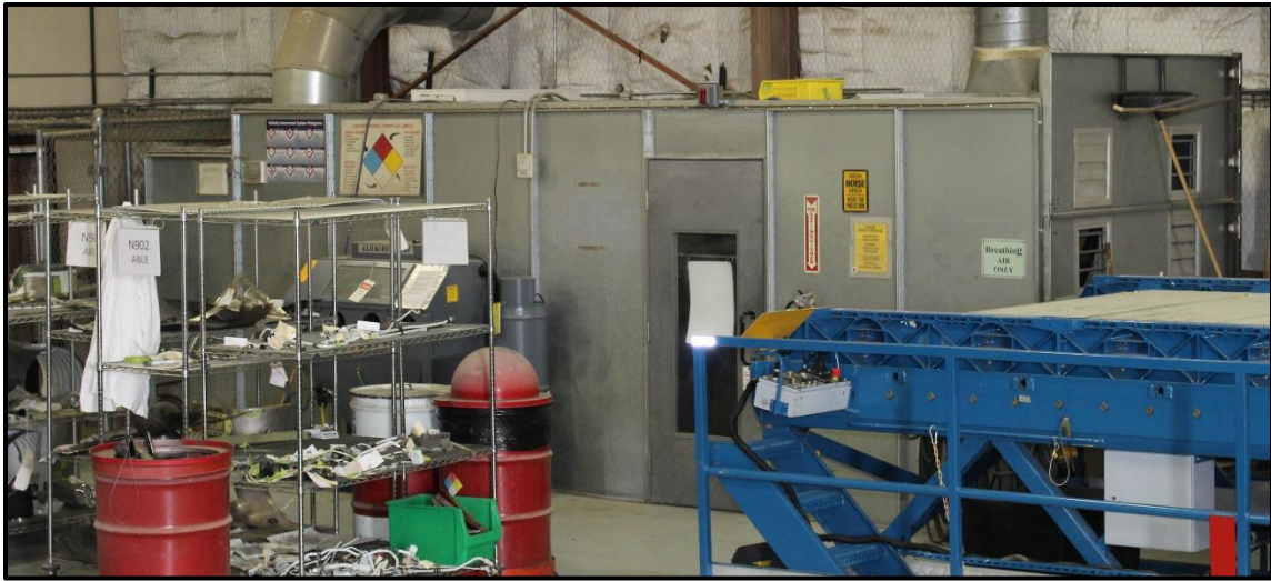
Figure 2-13. Ventilated Walk-in Booth Where Brakes Pads Are Replaced Photograph courtesy of NASA
