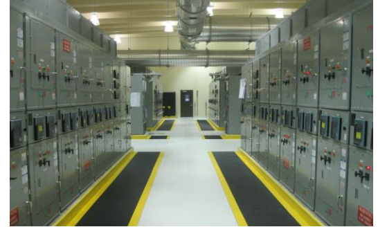
Electrical Distribution Site
