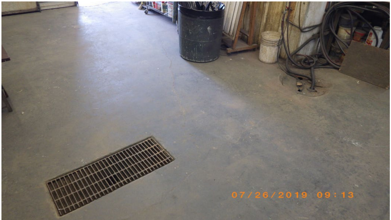
Figure 3 - Main Building Floor Sump
