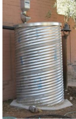
Figure 10: A cistern. (Source: Pima County and City of Tucson. Low Impact Development and Green Infrastructure Guidance Manual . March 2015.)
