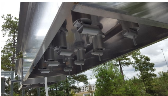
Figure 1. One of four sampling manifolds on the 32-cyclone collocated PE sampler at OAQPS in RTP, NC
