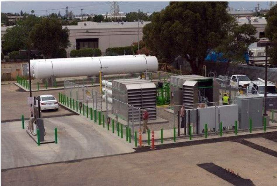
Figure 5.3 - RNG Vehicle Fuel Production and Fueling Facility
