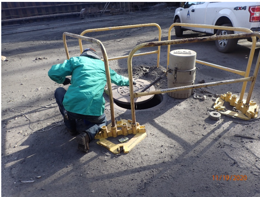
21: PB190021 Description: Taking a sample from sample location #01. Location: Storm Sewer Manhole #2316. Date/Time: November 19, 2020 10:06 A.M.
