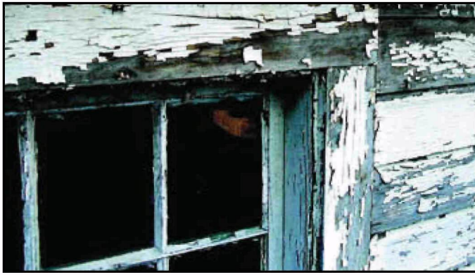
Figure 3-2. Chipping lead paint, which is a particular hazard to children when small particles are ingested.
