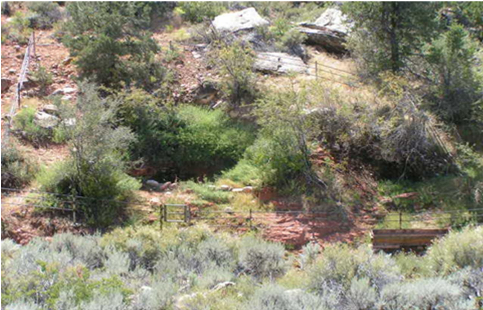
Section 319 Nonpoint source funds from EPA used to enclose Ridenour Spring, rock containment dam was constructed and plumbed to a wildlife drinker away and outside of the spring source; to prevent trampling of vegetation and to maintain water quality.
