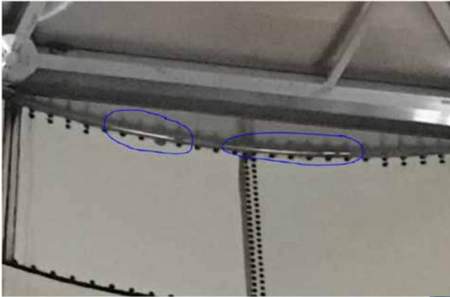
Unprotected openings in storage tank.
