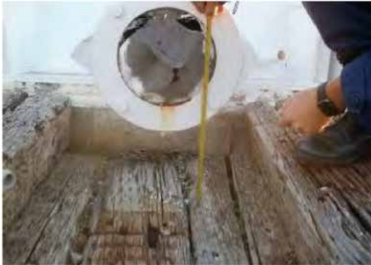
Overflow screening is torn and needs replaced
