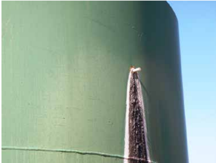
Un-repaired bullet hole in storage tank.
