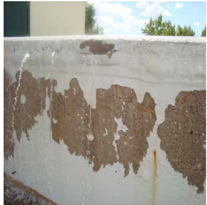
Leaking finished water storage tanks
