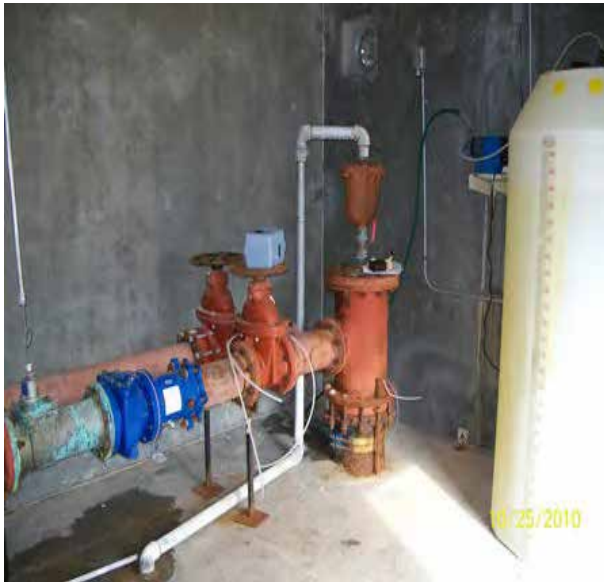
Cross connection with the venting/vacuum tied directly to the drain
