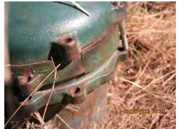
No wellhead sanitary seal; missing bolts = not properly sealed
