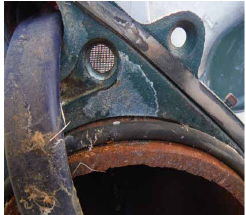
Lack of a sanitary seal
