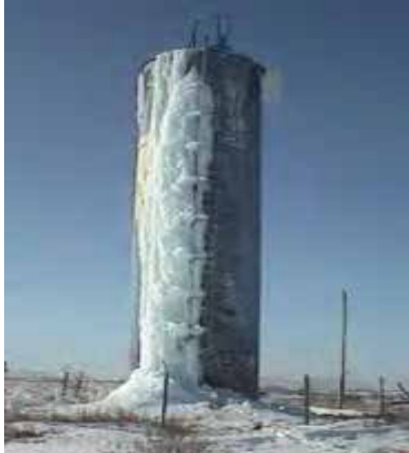
Frozen finished water storage tanks
