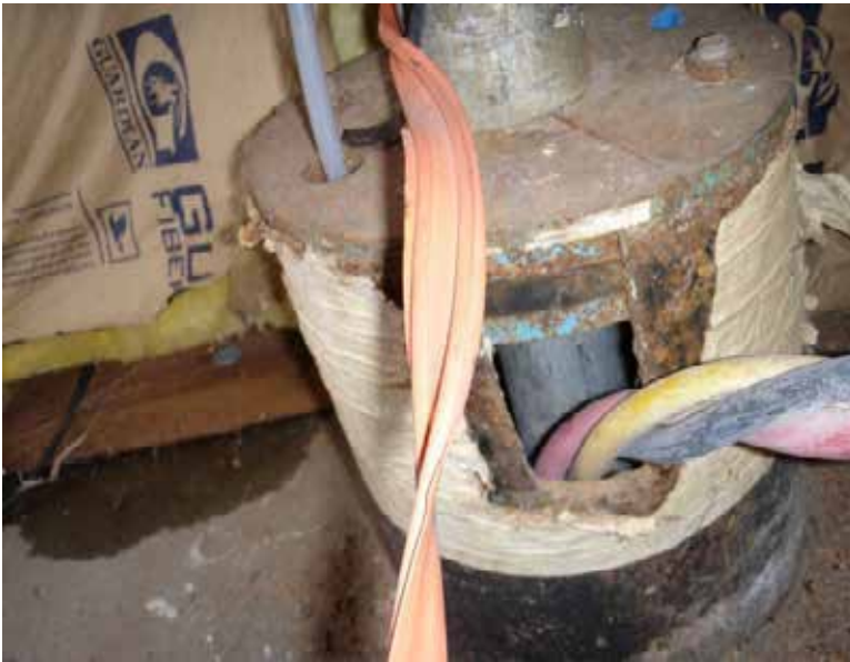
Conduit is not properly sealed.
