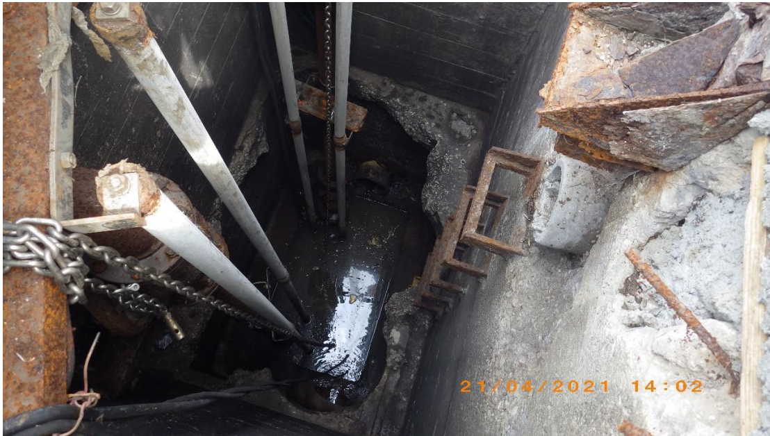
4: RIMG0098 Description: Falling Springs Lift Station – Wet Well. Location: 2897 Falling Springs Road Camera Direction: Down Date/Time: April 21, 2021 / 3:02 P.M.
