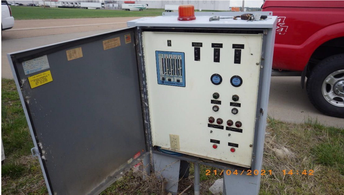
17: RIMG0111 Description: West #2-Bi-Grinder Station – Control Panel. Location: 1672 Sauget Industrial Parkway Camera Direction: Southeast Date/Time: April 21, 2021 / 3:42 P.M.
