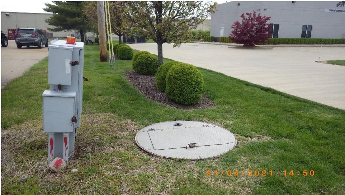
18: RIMG0112 Description: West #2-Bi-Grinder Station – Overview. Location: 1672 Sauget Industrial Parkway Camera Direction: Southeast Date/Time: April 21, 2021 / 3:50 P.M.
