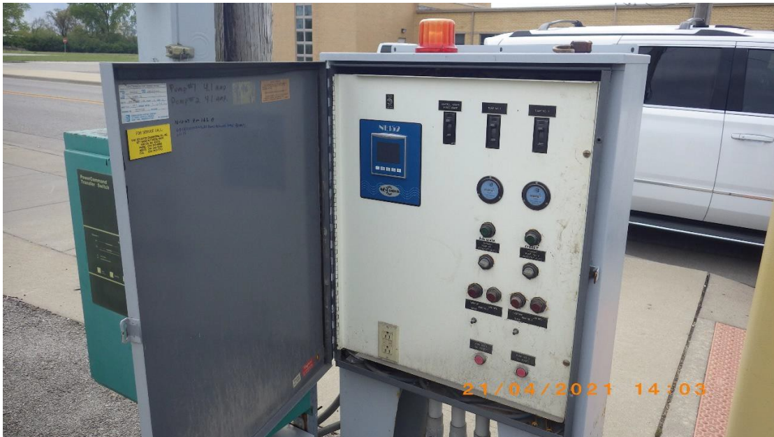
5: RIMG0099 Description: Falling Springs Lift Station – Control Panel. Location: 2897 Falling Springs Road Camera Direction: West Date/Time: April 21, 2021 / 3:03 P.M.
