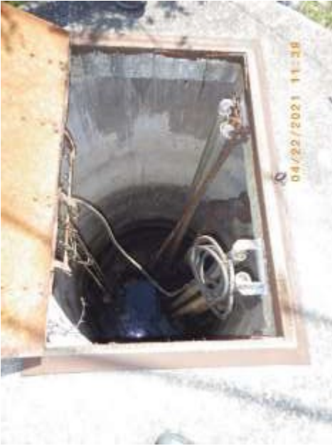
16: VCAH20006 Description: Lift Station #24. Location: Mississippi & David Camera Direction: 100° Date/Time: 4/22/21; 11:39 a.m.
