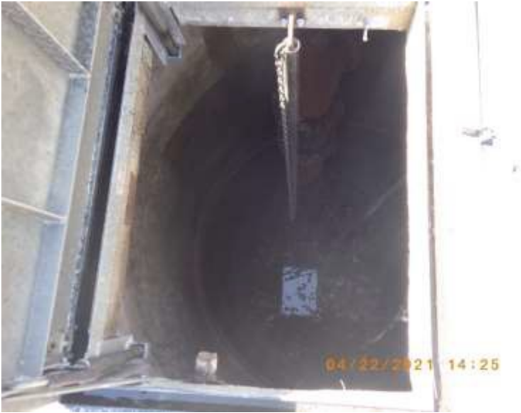
26: VCAH20016 Description: Lift Station #6, known as Cooper Station. Pump station. Location: Cooper & IL Rt 157 Camera Direction: 260° Date/Time: 4/22/21; 2:25 p.m.
