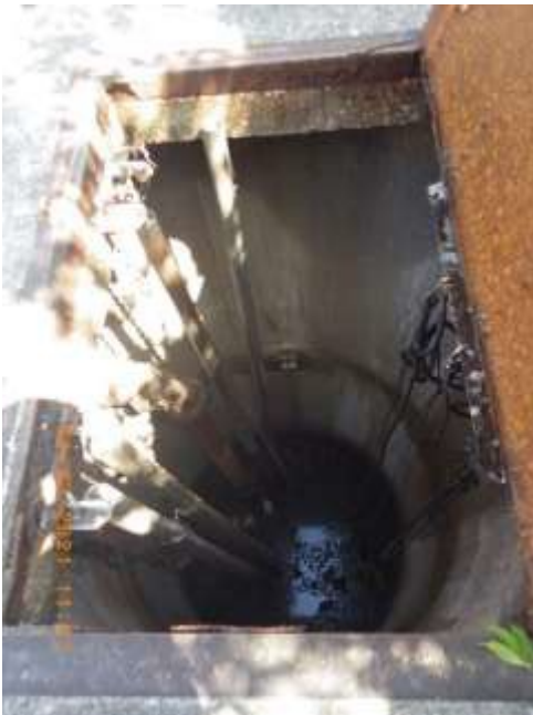
17: VCAH20007 Description: Lift Station #17. Note detached rail. Location: Mississippi & David Camera Direction: 19° Date/Time: 4/22/21; 11:47 a.m.
