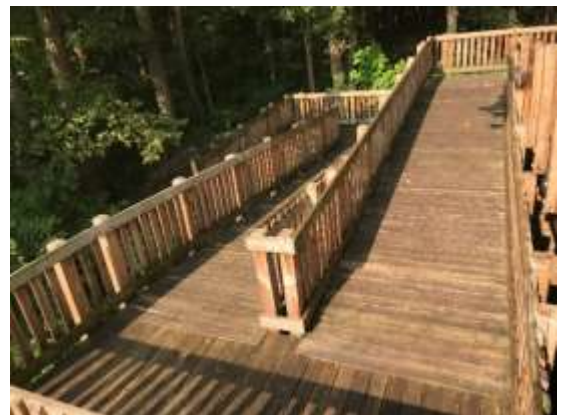
TCWP partners worked to improve a bridge over Trail Creek, connecting the Karwick Nature Park and the Cheney wetland project.
