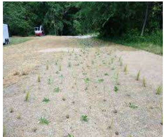
LaPorte County Parks installed a bioswale to intercept parking lot runoff at Creek Ridge Park.
