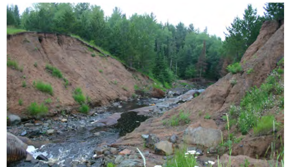
► The 2012 event also overtopped a 200 foot culvert. © Fond du Lac Resource Management Division
