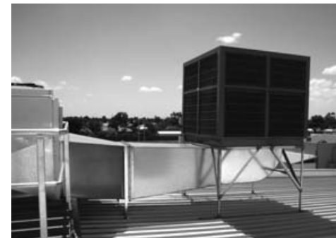
Figure 5: Evaporative cooling module
