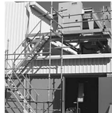
Figure 1: The propylene chiller on the roof and the CO 2 unit in the room under during commissioning
