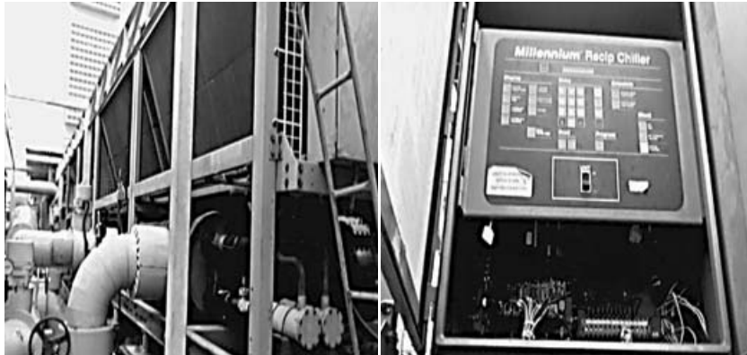
Figures 2 and 3: Far East Square Shopping Complex, Roof Top, Chiller No 3, York Air-Cooled System Model: YDAJ98MU7-50PA
