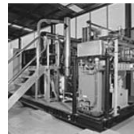
Figure 6: CFC, HCFC, HFC and halon destruction system
