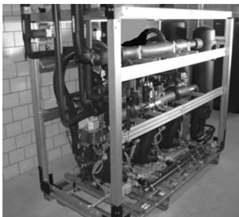
Figure 9: Picture of the LT unit with two-stage compression and two-stage throttling
