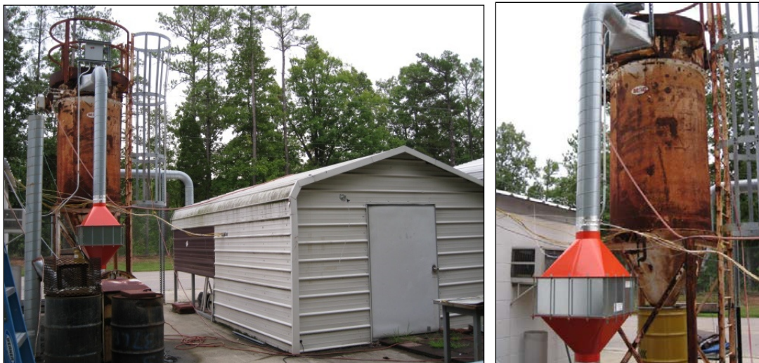
Figure 3-5. Burn Hut, Baghouse, and HEPA Filter.
