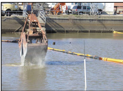
Sediment capping at the Anacostia River Watershed in the District of Columbia.
