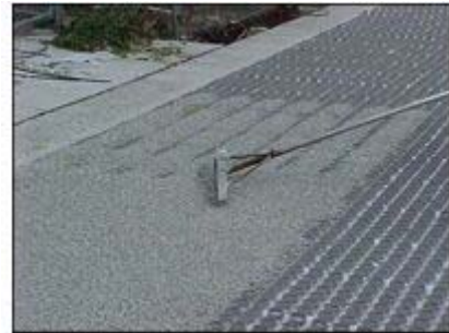
Raking gravel into a Gravelpave2 system (courtesy of the City of Chicago).
