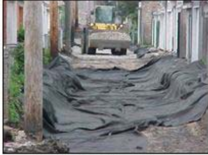
Making way for a porous pavement alley (courtesy of the City of Chicago).
