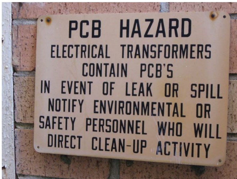
Sign at P&W Waste Oil Services, Inc. located next to the transformers where the PCB oil was removed.
