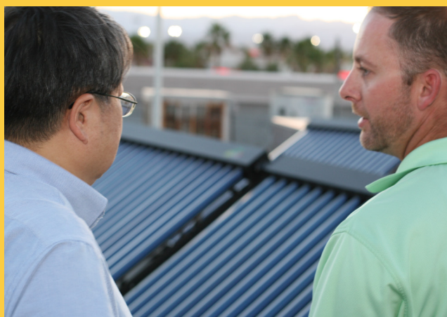
Dave Zheng (left) inspects the new solar hot water system with a member of his installation crew.
