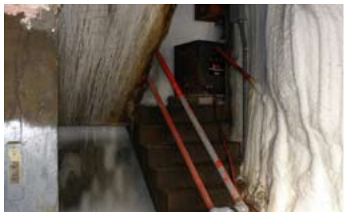
Ice Buildup Blocking Stairway
