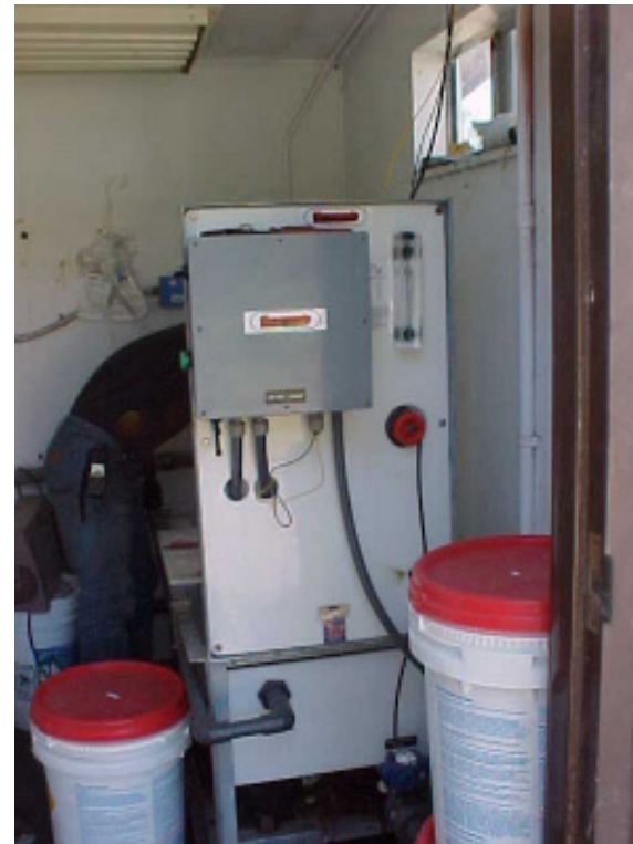
A Chlorination System
