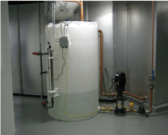
Condensate holding tank with piping, GSA Metcalfe Federal Building in Chicago.
