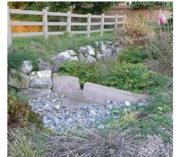
Cascading (terraced) bioretention cells in Seattle are separated by notched concrete weirs.
