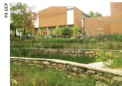
Adding structural walls to this terraced treatment train allowed it to be built in a sloped area.
