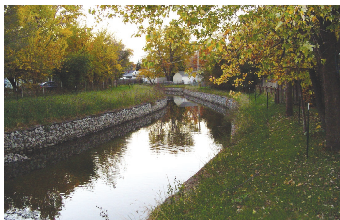
Figure 2. A gabion toe (cage filled with earth and rocks) protects the left and right banks in this section of Addison Creek.
