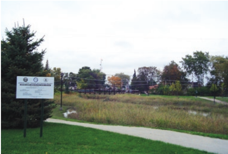
Figure 4. Along this section of the creek, the partners restored a streamside wetland and stabilized the streambank with vegetation, riprap, and riffles.
