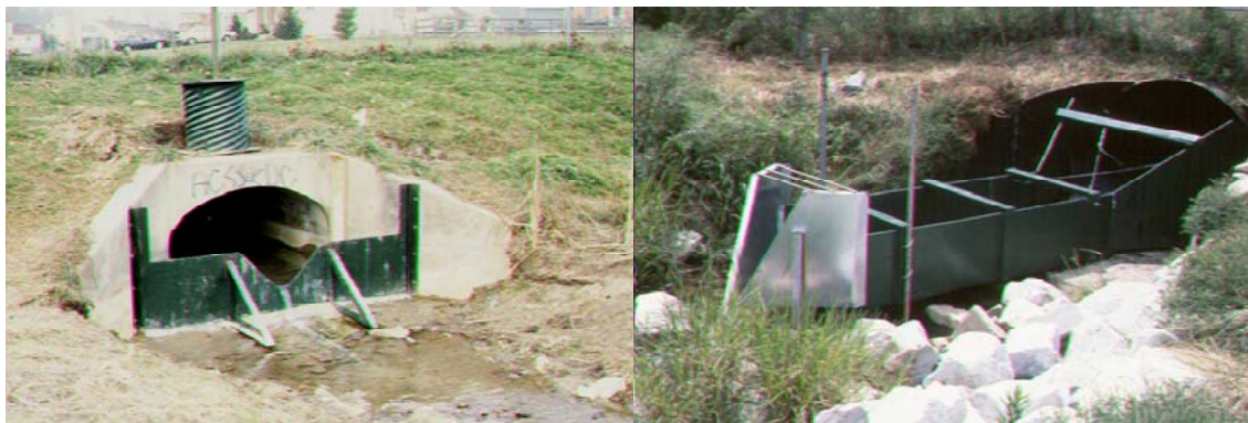
Figure 1. Example outfall monitoring with V-notch weir and flume set-up. (photo courtesy City of Baltimore, MD)
