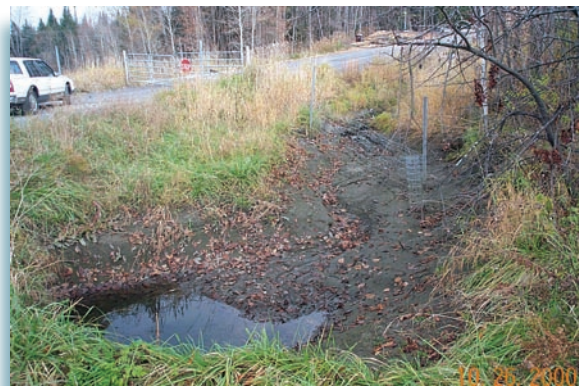
Ditch near Adams Brook prior to being lined with rock. Rock lining reduced sedimentation into Adams Brook.
