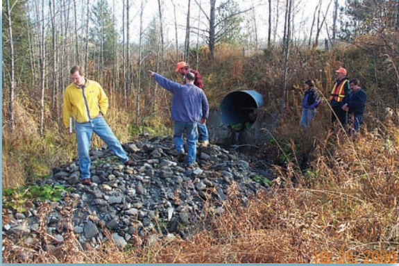
Geomorphic instability and an unauthorized culvert (upstream of the location in this photo) caused heavy erosion and the dumping of rock piles at the culvert shown here. Removing the unauthorized culvert helped to address the instability and reduce the water quality impacts on Adams Brook.
