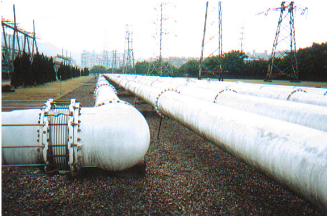
GIL(Gas Insulation Line)
