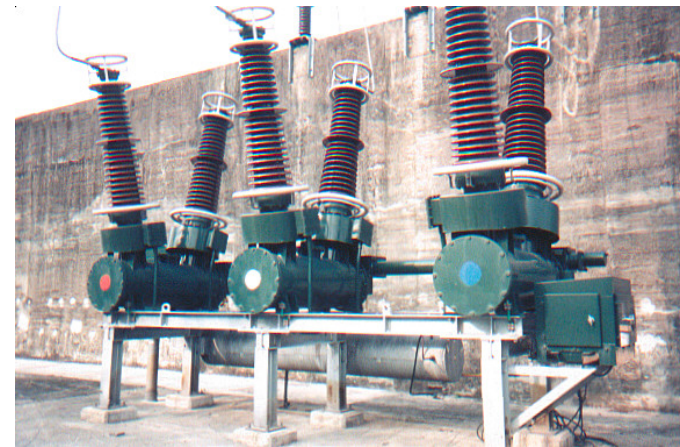
GCB(Gas Circuit Breaker)
