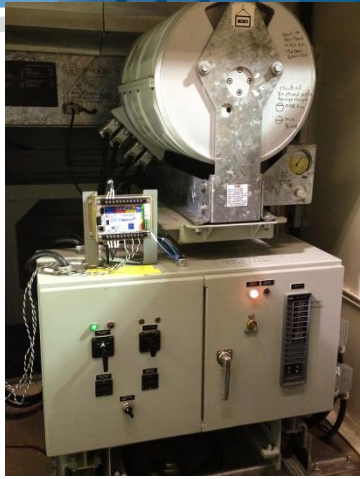
Pumped-Storage Generator Breaker
