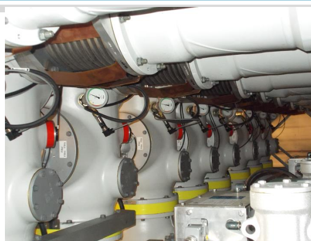
GIS Circuit Breakers & Sections
