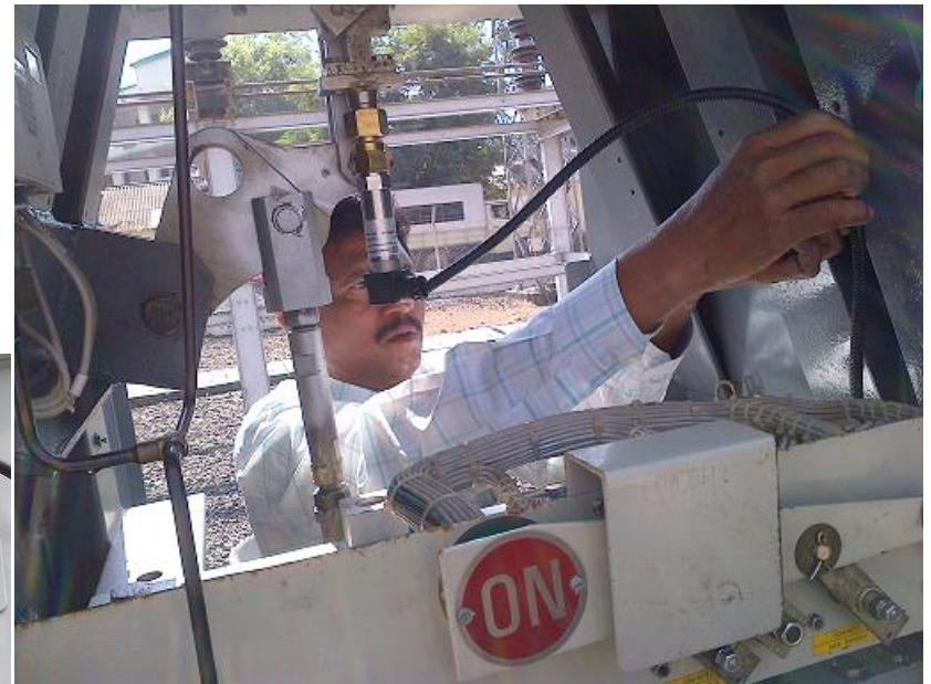
Crompton-Greaves 245kV Live Tank
