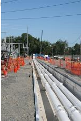
SF 6 Insulated Bus
