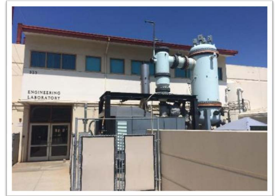
Ener-Core Powerstation at UC Irvine Campus
