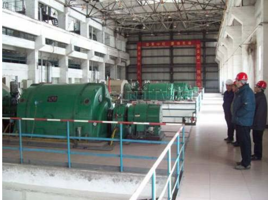
Figure 1.11: 6-MWe Steam Turbine in Coal Fired Power Plant in Erdoaling Area
