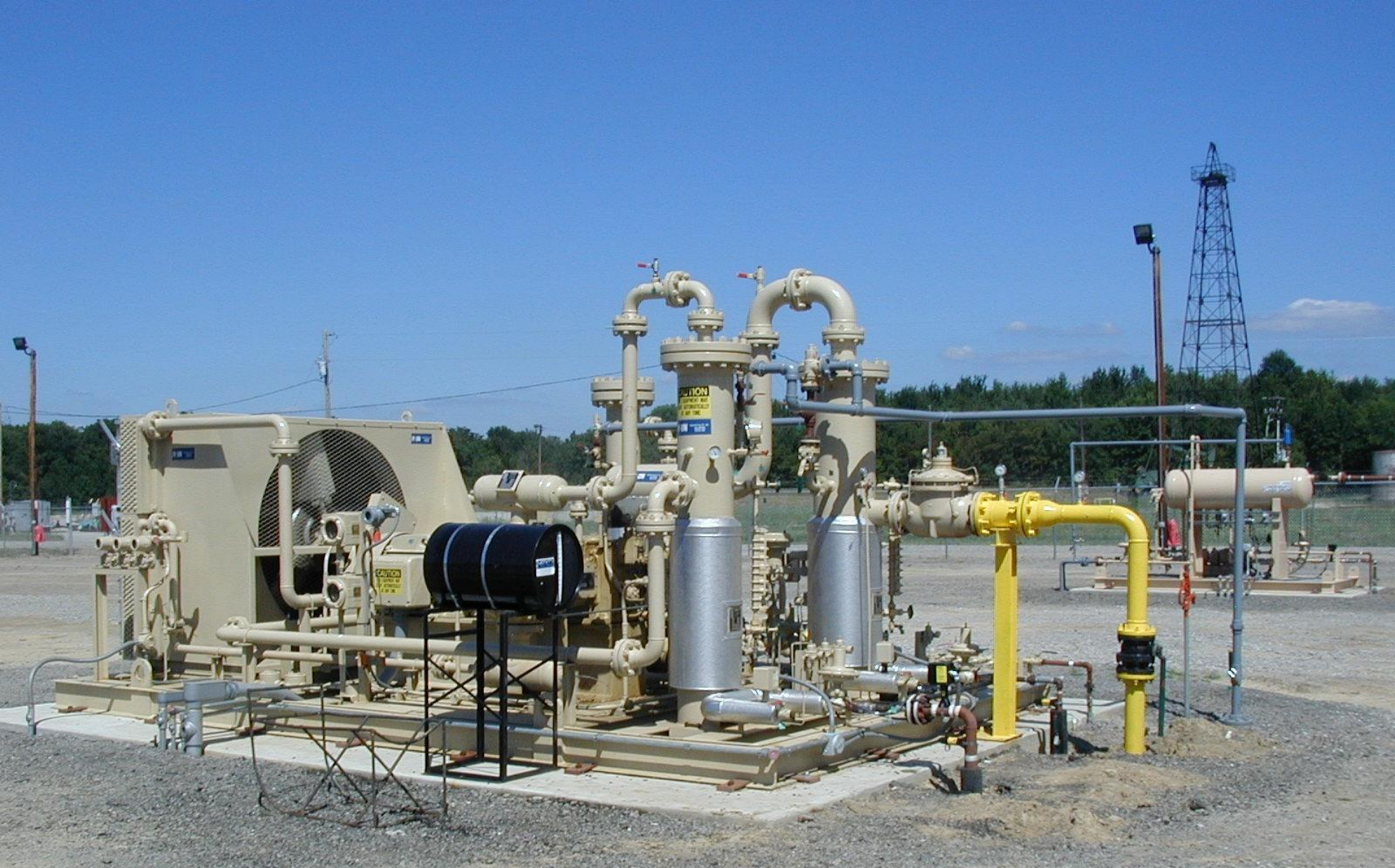
Plant Compressor (Boosting gas to Salem)
