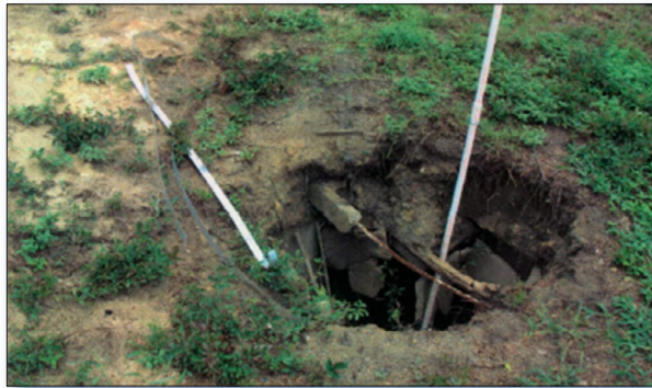
Figure 2. This Horse Creek watershed septic system had failed due to a cave-in.
