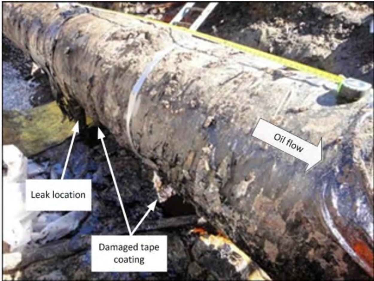
Figure 3. View of the damaged tape coating on the oil pipeline in the excavated trench
