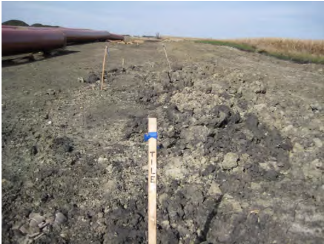
Figure 7: Tile damaged, water courses changed (sidewall compaction, channel change, ...). Enbridge knew there was tile there. Tile not repaired, new tile over pipe crushed on backfill of trench.
