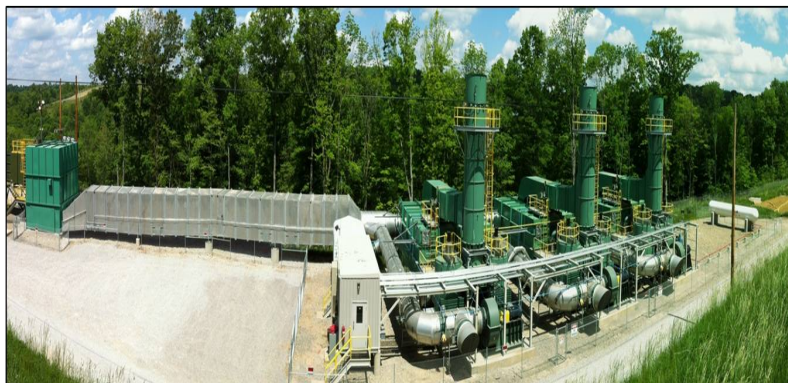
Verdeo McElroy VAM Abatement Project, Marshall County Mine, West Virginia, USA (courtesy of Sindicatum Sustainable Resources)
