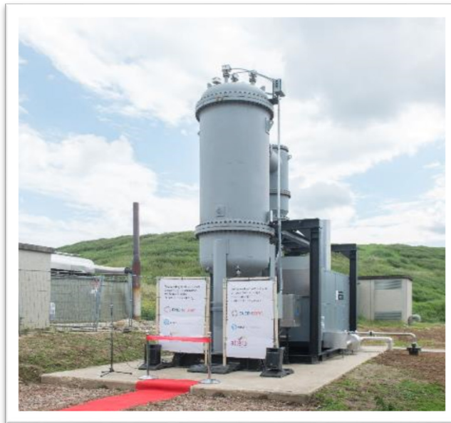
Ener-Core Powerstation EC250 (courtesy of Ener-Core, Inc.)
