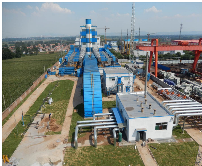
Fortman Clean Energy Technology Ltd VAM Abatement Project, Gaohe Mine, Shanxi Province, China (courtesy of Dürr Systems)
